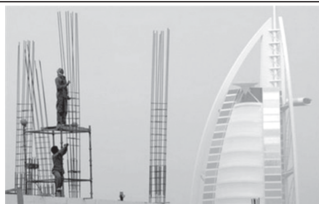
Foreign labourers work at a construction site in front of Dubai's landmark Burj al-Arab hotel on 22 March. Faced with a sudden economic slowdown, Dubai is trying to combat the fraud cases that surged during the past years of rapid economic growth in a bid to boost its status as a regional business hub. —INTERNET
