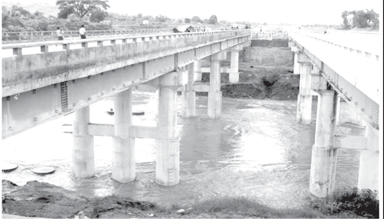
The 360-foot long Tonkan Bridge near Mile Post No 93/2 on Yangon-Nay Pyi Taw Road.
