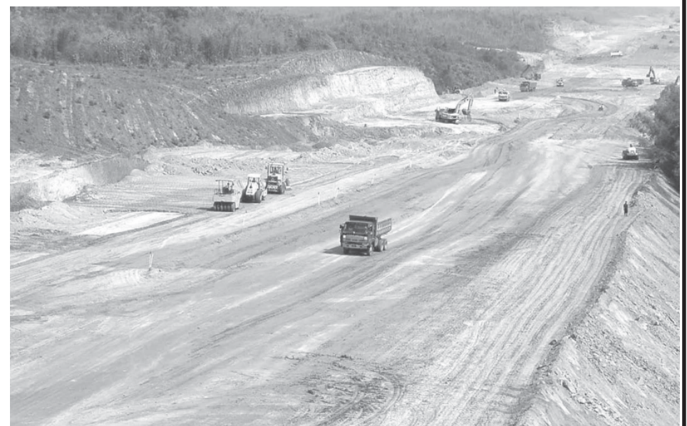
Land preparations on construction of Nay Pyi Taw C Junction-Pantin section near Mile Post No 210.
