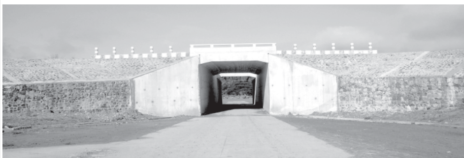
Photo shows underpass near Mile Post No 83/6 on Yangon-Nay Pyi Taw Road Section.
