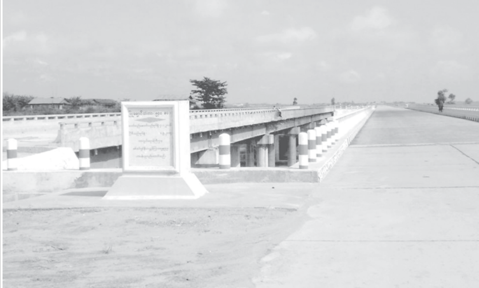
The 540 feet long Pyu Creek Bridge under construction between mile post No 114/0 of Yangon-Nay Pyi Taw road section.
