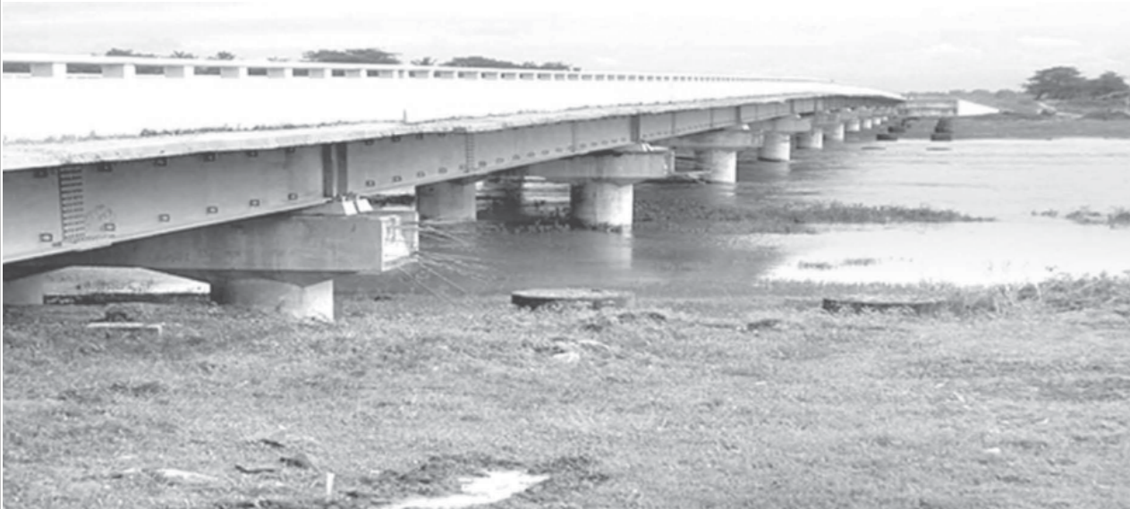
The 990 feet long Khabaung Bridge near mile post No. 144/6 of Yangon-Nay Pyi Taw road section.
