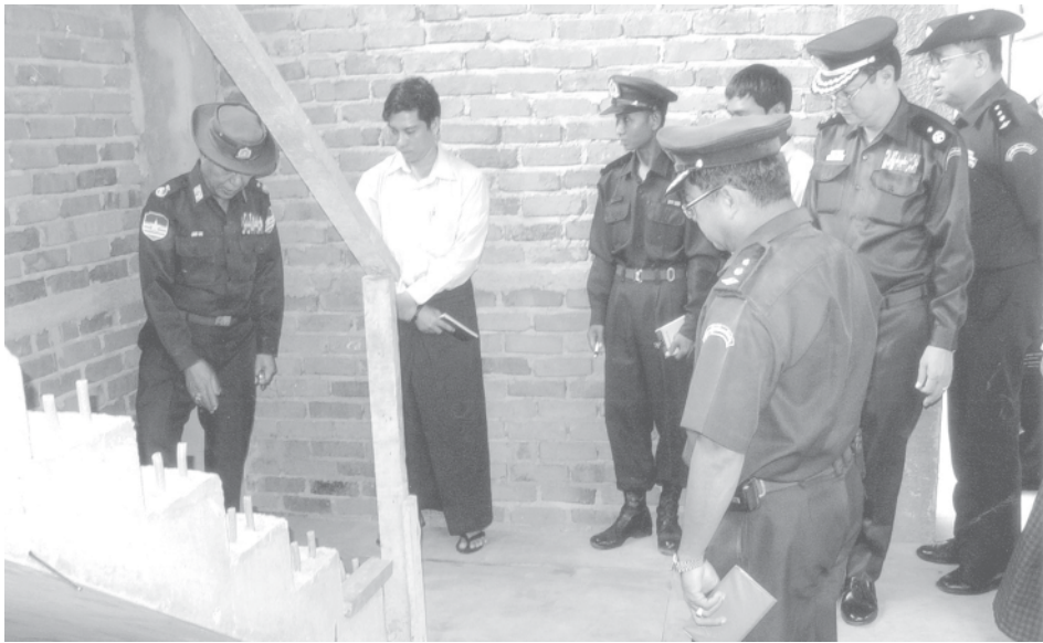
Minister Maj-Gen Maung Maung Swe inspects fire station under construction in Kawhmu Township, Yangon Division.—FSD
