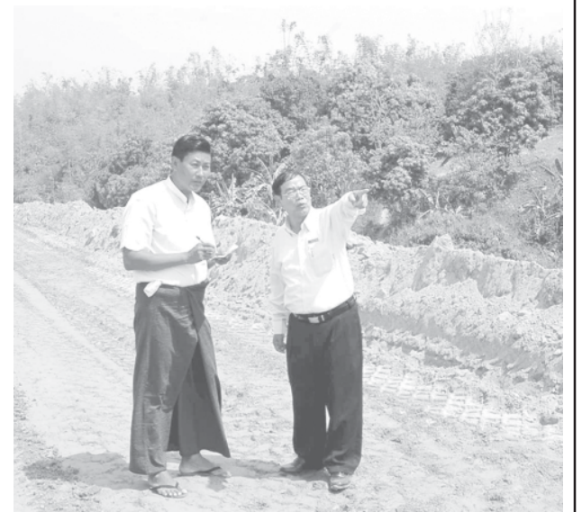
Project Engineer U Tint Hsan explains process of filling 80 to 100 feet deep ravines and gorges with earth.
