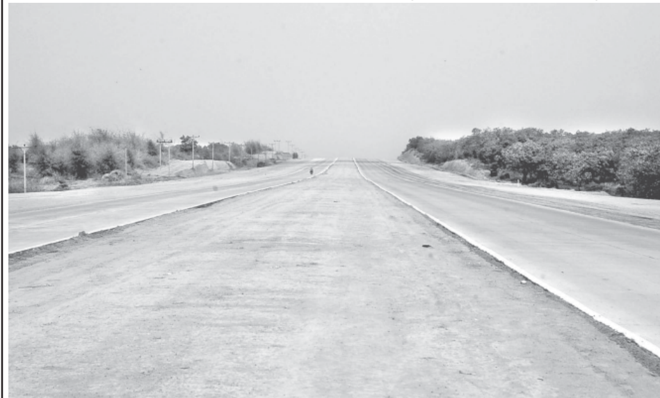
Progress in constructing the two-way / two-lane concrete road between mile post Nos 26/4 and 83/6 of Yangon-Nay Pyi Taw road section.—MNA
