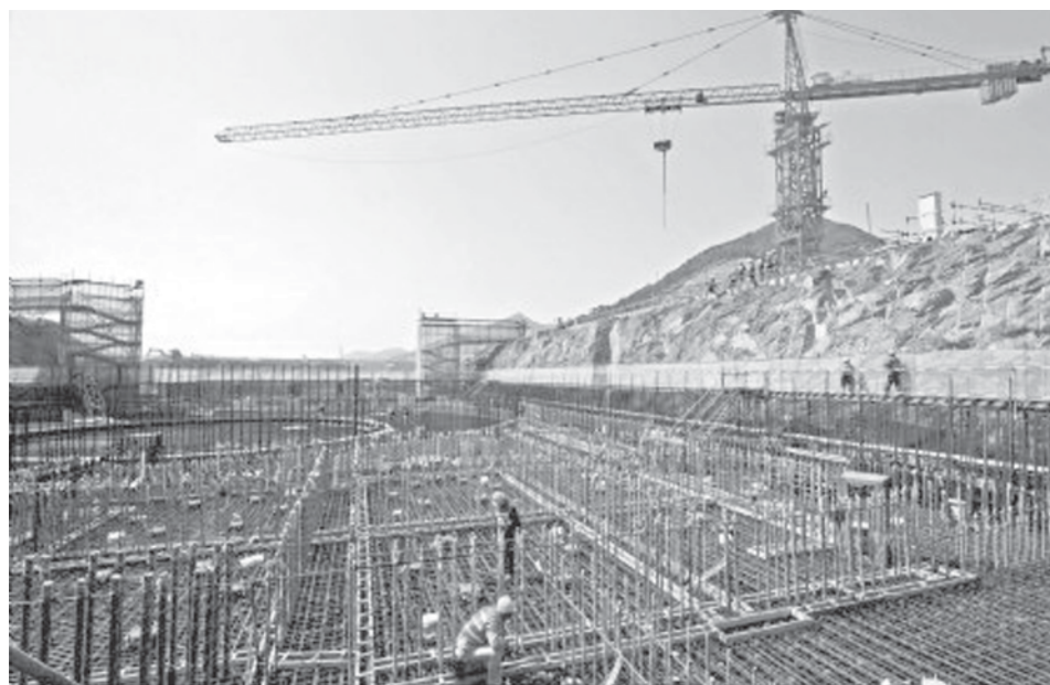
Picture taken on March 15, 2009 shows a construction site of the Sanmen Nuclear Power Project (NPP) in east China's Zhejiang Province. The first phase of the Sanmen NPP is now ready for startup.—INTERNET
