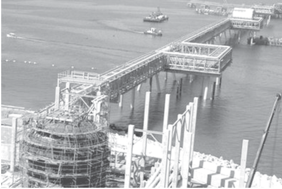
A part of Yemen's second liquid natural gas plant is seen under construction in the coastal area of Balhaf, southeast of the capital Saana. Yemen, one of the poorest countries on Earth despite its proximity to oil powerhouse Saudi Arabia, hopes to join the international club of gas exporters this year — and reap a desperately needed multi-billion dollar windfall.—INTERNET
