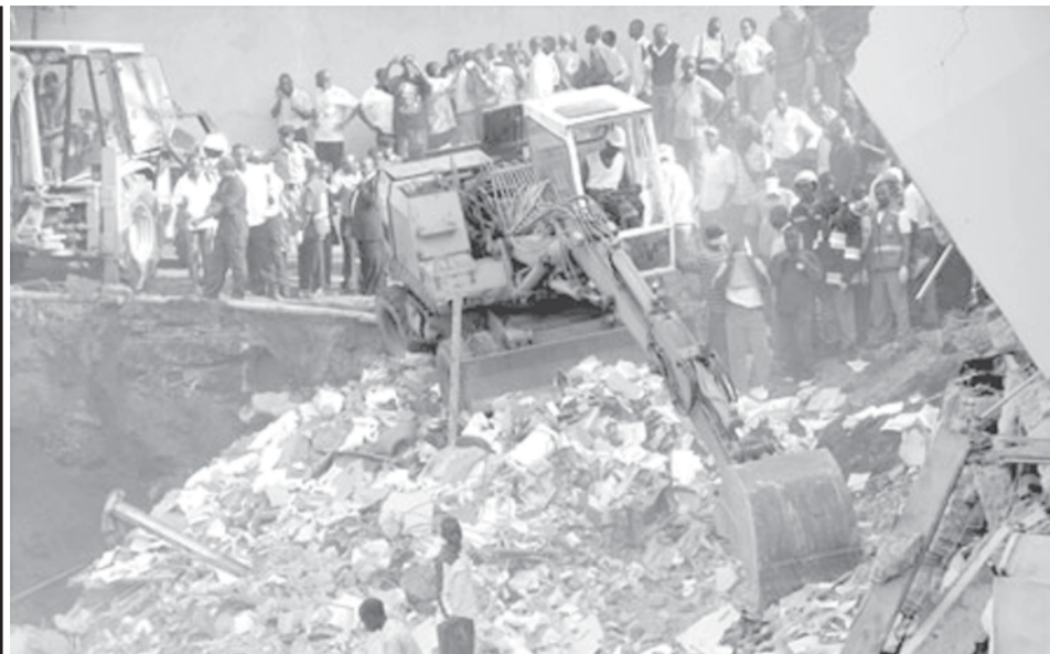
Rescuers work at the site of a collapsed building on Nasser Road in downtown Kampala, Uganda, on 13 March, 2009. A two-storied shopping arcade collapsed Friday afternoon after a nearby construction loosened its foundation, two people have been confirmed killed. Judith Nabakooba, the police spokesperson, told Xinhua that another seven were injured while an unknown number of people were still trapped in the rubble.—XINHUA
