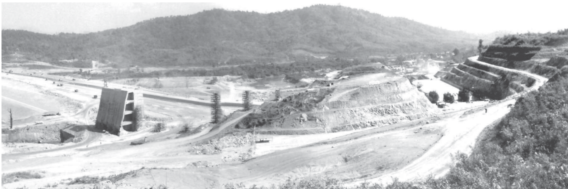
The worksite of Shwegyin Hydropower Project, about six miles northeast of Shwegyin.
