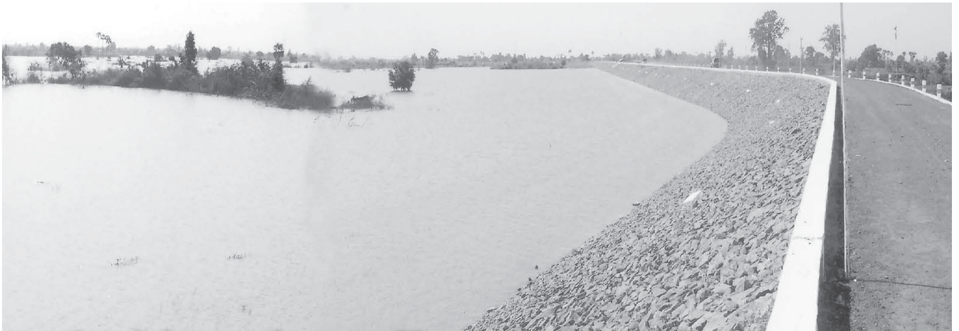
Photo shows storage of water at Paygyi Dam in Kanbalu Township, Shwebo District.
