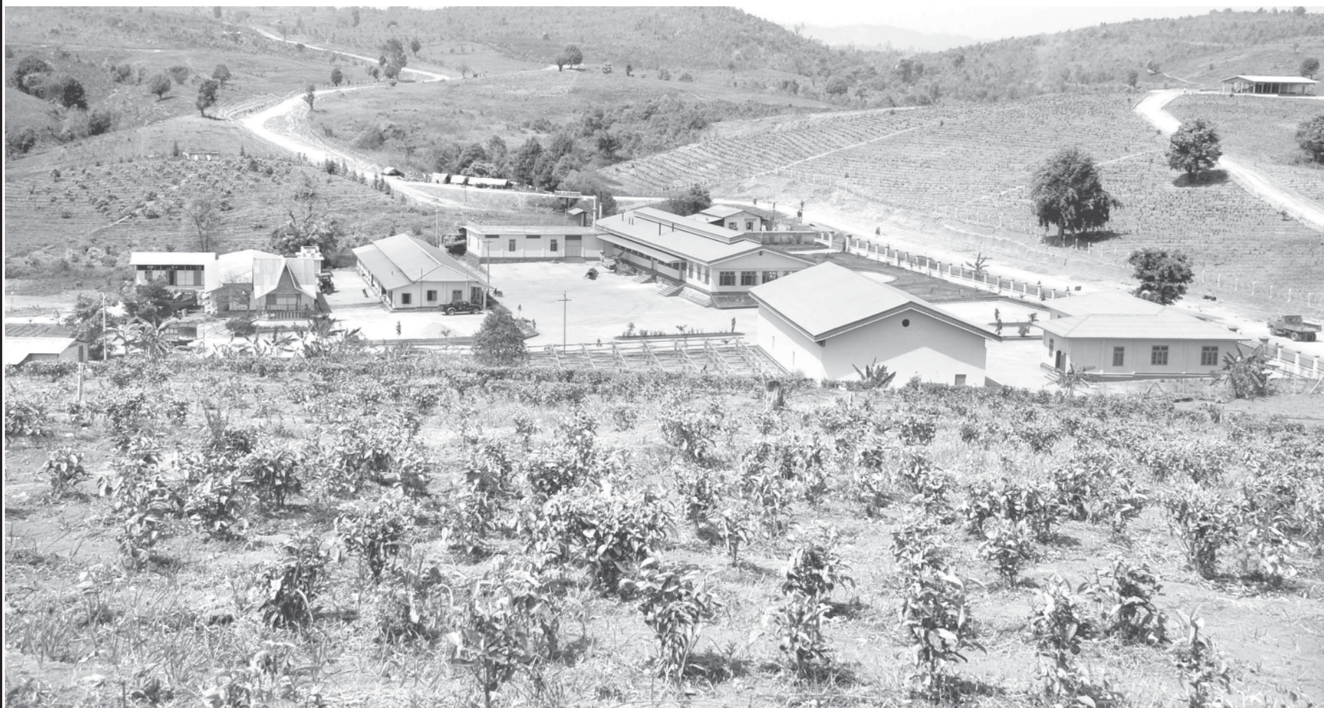
A tea factory under construction near Khoyawng Village-tract, Tangyan Township, Lashio District.
