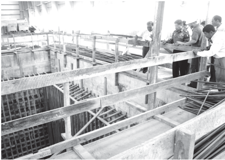
Industry-2 Minister Vice-Admiral Soe Thein inspects completion of machine foundation of 16-ton Press Machine at Forging Shop.
