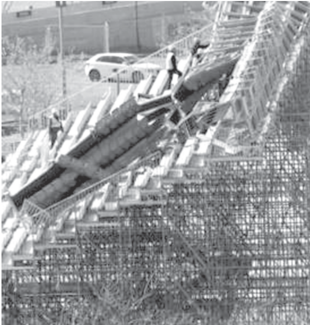
Technicians inspect damaged spectator stands due to high winds on the top of a purpose-built arena for the Spain's Davis Cup match against Serbia in Benidorm on 6 March, 2009. The tie has been suspended due to high winds as the weather conditions had made the purpose-built arena on the outskirts of the seaside town unsafe, the Spanish tennis federation (RFET) said on Friday.—INTERNET
