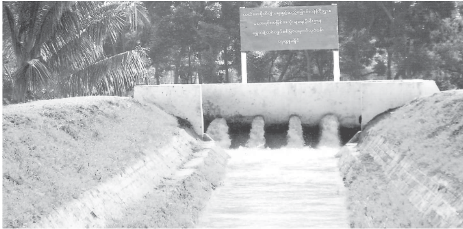
Shwetanttit pumping station providing irrigation water for over 5,000 acres of farmland near Shwetanttit Village of Pakokku District.
