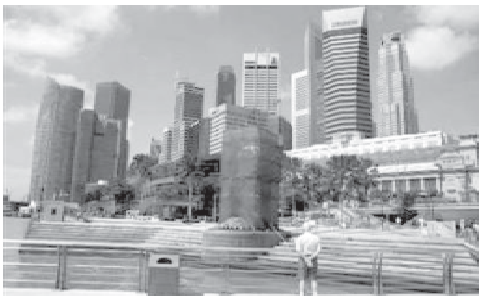
A tourist looks at the covered Merlion statue as it undergoes repair in Singapore on 2 March, 2009. Singapore's iconic Merlion statue, a popular tourist attraction, was damaged by lightning on Saturday afternoon during a thunderstorm, government radio reported.—INTERNET
