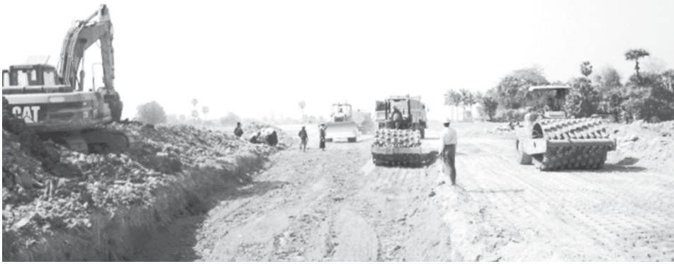
Road works in progress at mile post (142/6) on Myochaung-Thagara road section. —MNA
