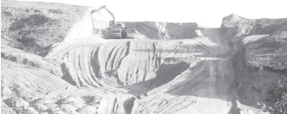
Earth works in progress at mile post (230/1) on Pantin-Paybinlay-Kukwe village road section. —MNA
