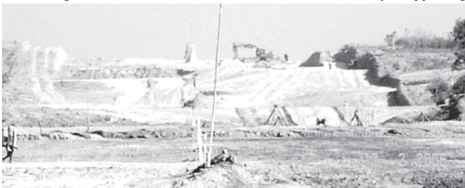
Earth works in progress at mile post (119/0) on Myochaung-Thagara road section. —MNA
