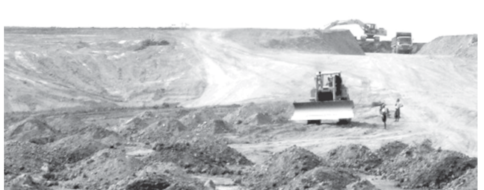
Earth works in progress at mile post (246/4) on Pantin-Paybinlay-Kukwe village road section. —MNA
