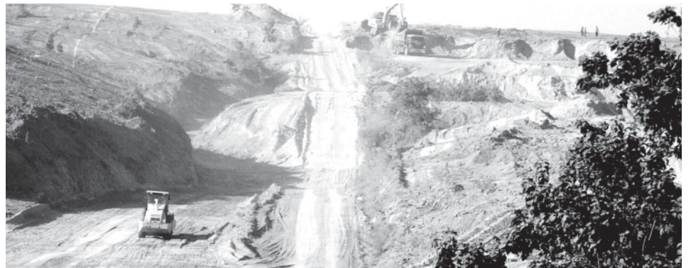
Earth works in progress at mile post (237/4) on Pantin-Paybinlay-Kukwe village road section. —MNA
