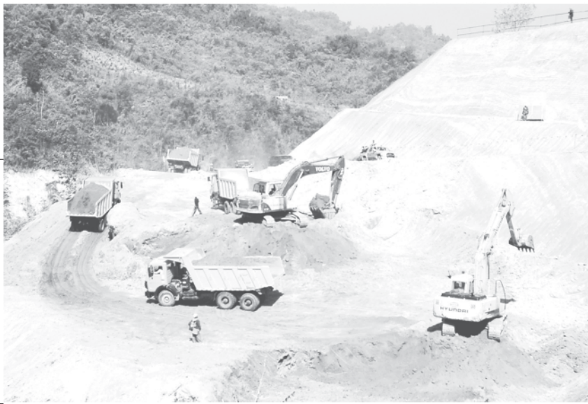
Maj-Gen Ohn Myint of Ministry of Defence inspects construction of embankment and intake canal of Chipwenge Hydro Power Project.—MNA
