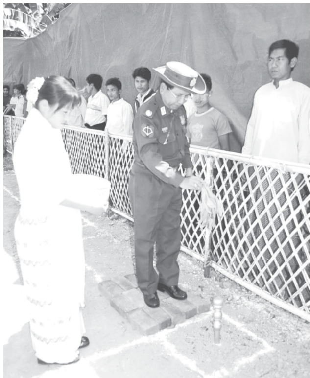
Minister Brig-Gen Kyaw Hsan drives stake for construction of library in Nanchaung village of Thandwe Township.—MNA
