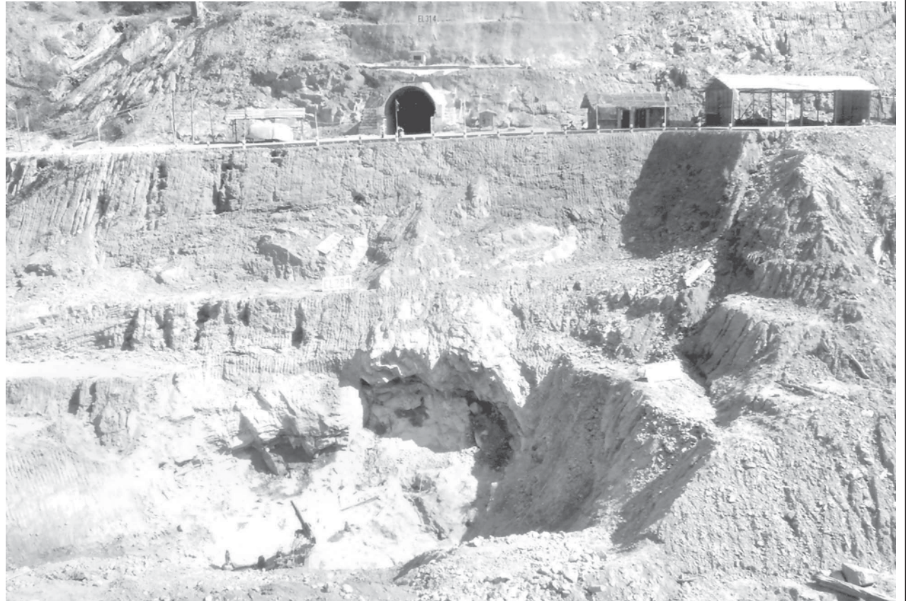
Photo shows land preparations at Salu Creek for building concrete posts of the bridge for intake tunnel and aqueduct.
