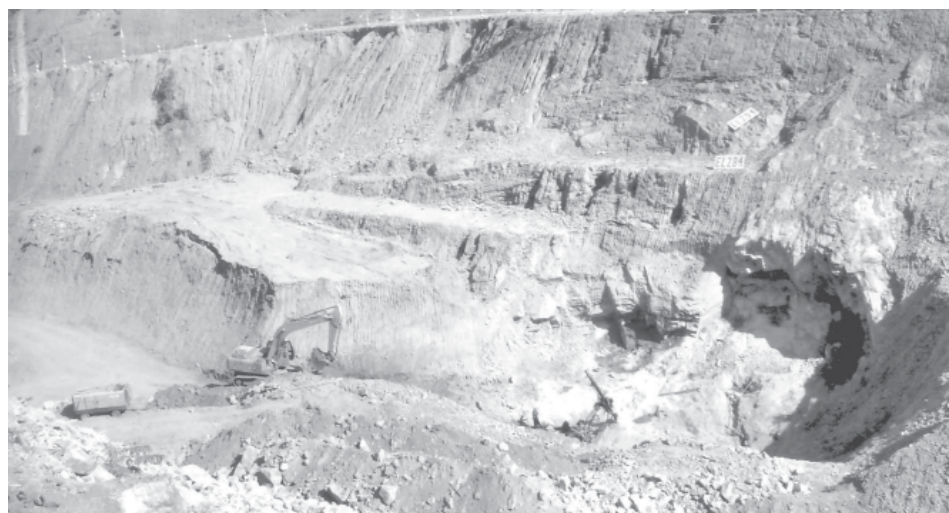
Ground preparations being made for construction of concrete posts at Salu Creek.
