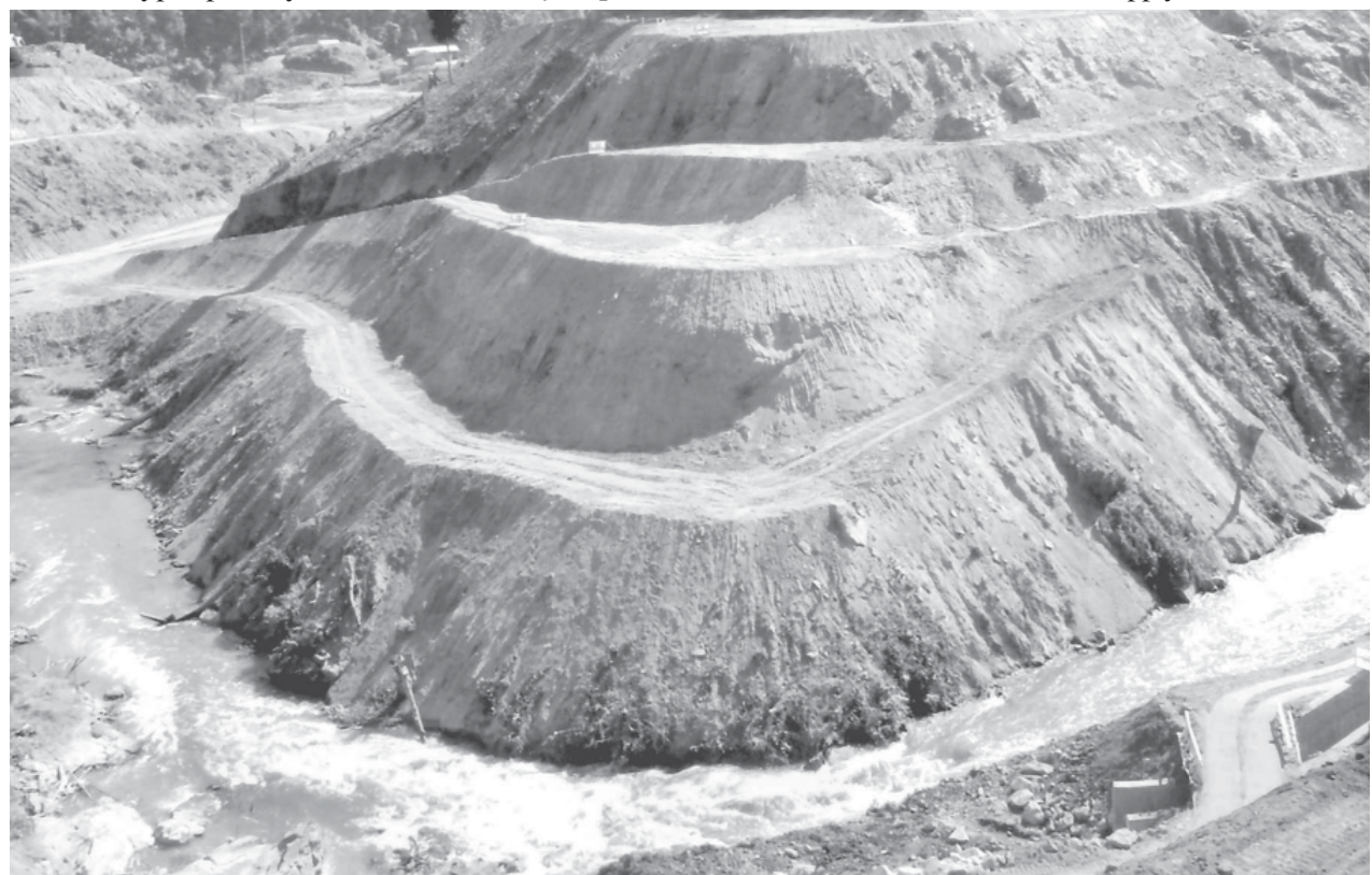
An aerial view of Nancho Creek and construction site of Nancho Hydropower Plant.
