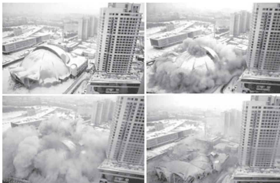
A combination of photographs shows a water amusement centre called "The Summer Palace" falling in a demolition blast in Shenyang, Liaoning Province, on 20 Feb, 2009. The landmark dome structure was dismantled to make way for construction of a new property development after serving 15 years as a fun place for local residents.—XINHUA
