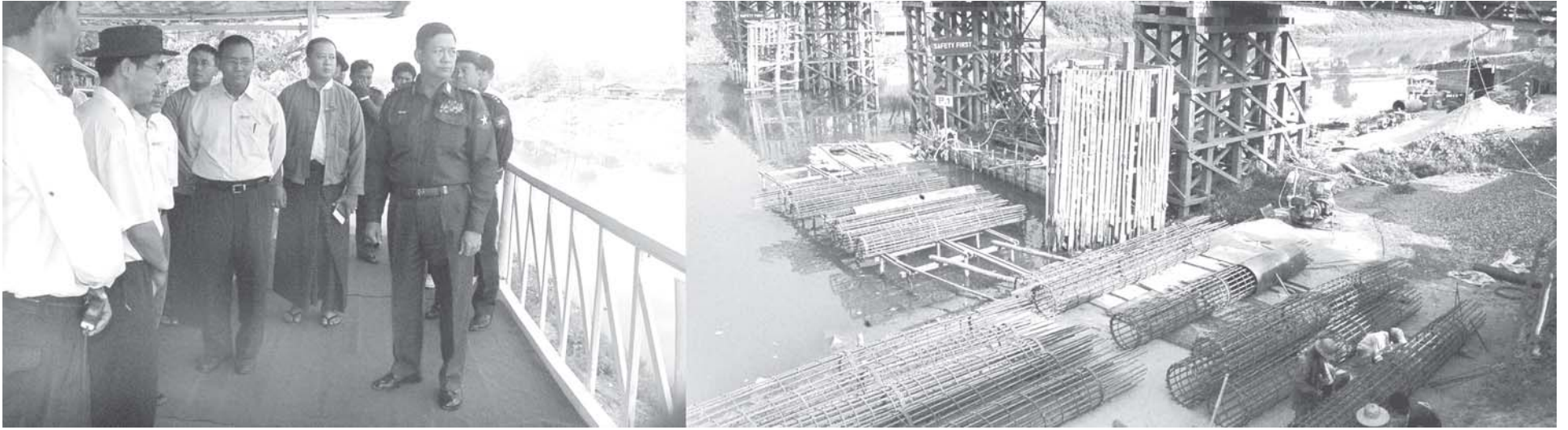
Maj-Gen Ko Ko of Ministry of Defence inspects under construction of Bago Bridge project in Bago Township.—MNA
