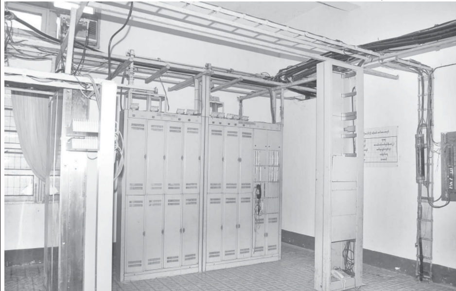
Control room of communication station in Mon State.
