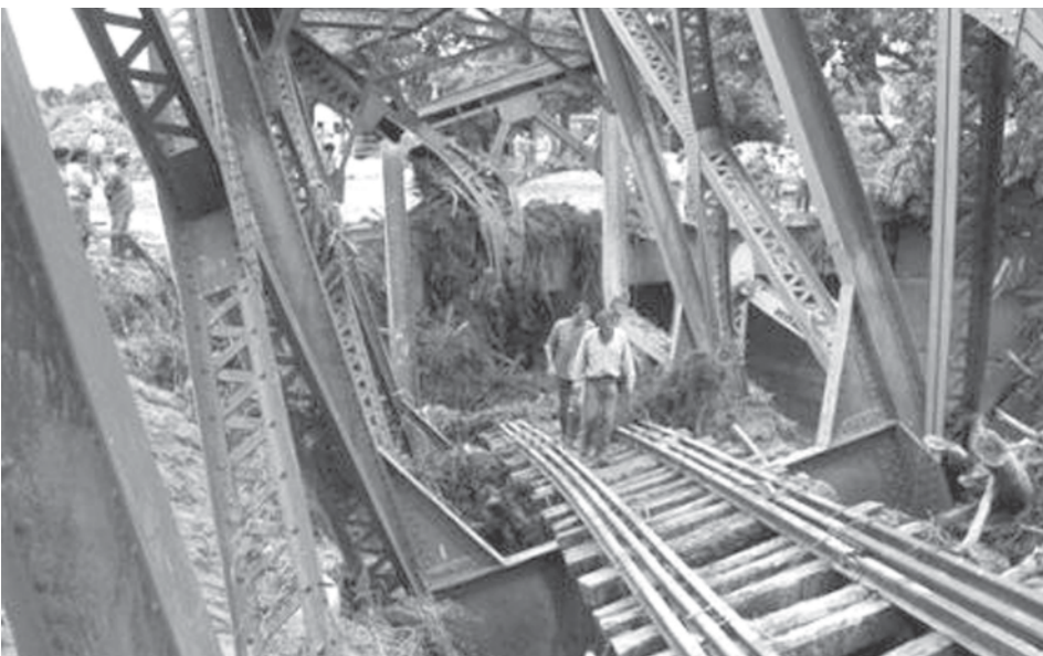
People walk on a bridge destroyed by a landslide in the northern Argentine city of Tartagal on 10 Feb, 2009. —INTERNET
