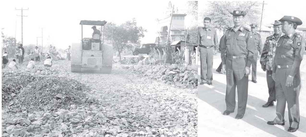
Maj-Gen Ohn Myint of Ministry of Defence inspects upgrading of roads in downtown Mandalay.—MNA
