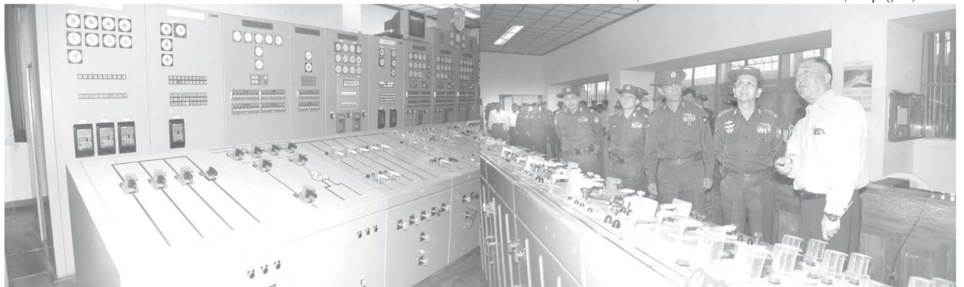
Prime Minister General Thein Sein visits control room of Biluchaung No. 2 Hydropower Plant.—MNA
