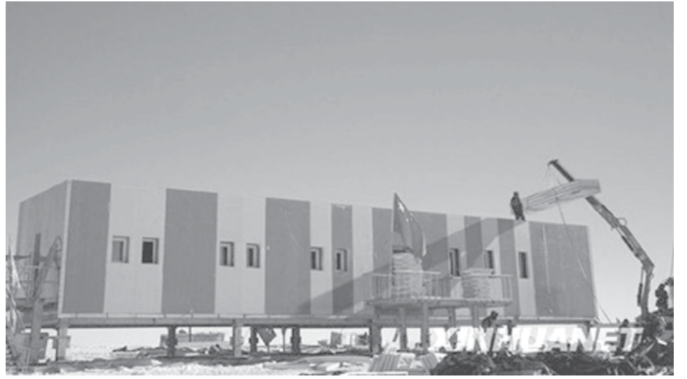
Photo shows the Kunlun Station under construction. China set up the country's third Antarctic research station on recently. —XINHUA
