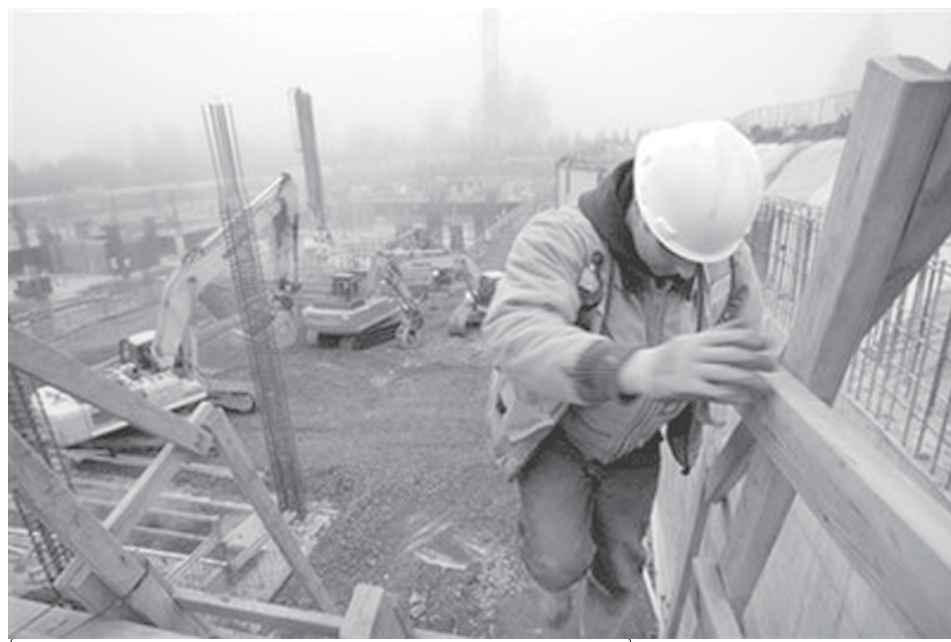
A worker climbs into a giant pit at a construction site on the Microsoft campus that is expected to be delayed or halted, in Redmond, Washington. The economy shrank at a 3.8 percent pace at the end of 2008, the worst showing in a quarter-century, as the deepening recession forced consumers and businesses to throttle back spending.—INTERNET
