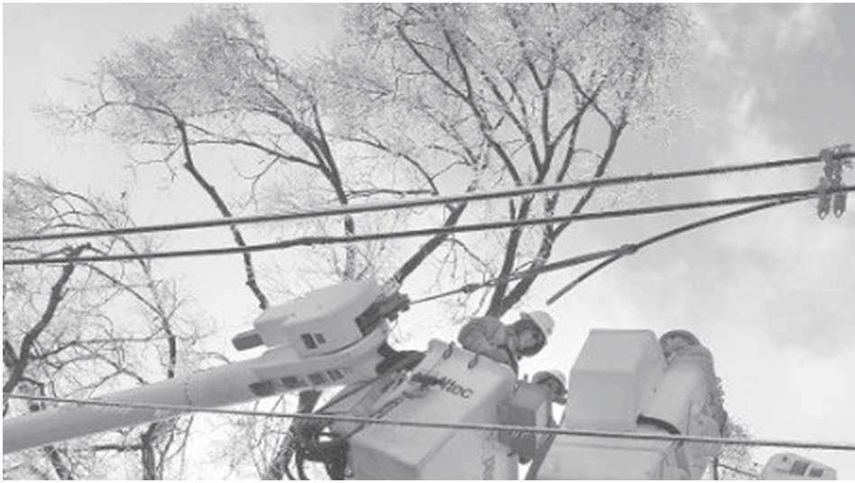
Linemen work to restore electricity to more than 200,000 Louisville residents, days after an ice storm hit the city on 30 Jan, 2009. More than 600,000 homes and businesses were still without power on Friday morning after snow and ice storms earlier this week left more than 1.5 million customers in the dark from Oklahoma to Pennsylvania, local utilities reported. The storms on 27-28 Jan, hit Kentucky the hardest, leaving more than half a million customers without power.—XINHUA
