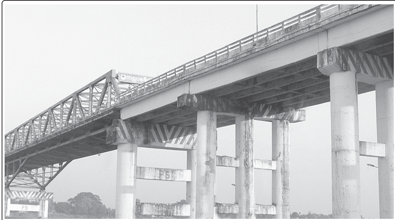
Well-known Kissapanadi Bridge lies on Yangon-Sittway Road linking MraukU and Kyauktaw in Rakhine State. (See page 7)
