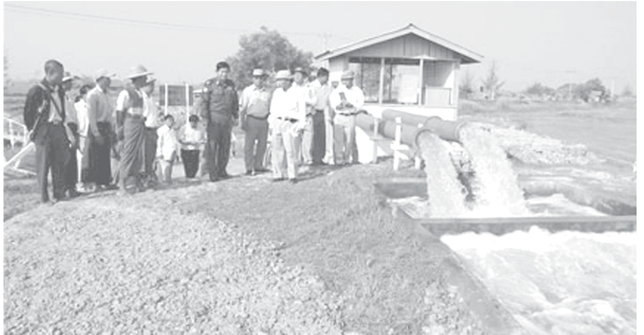
Minister Maj-Gen Htay Oo inspects Malit River Water Pumping Project in Hlegu Township.—MNA
