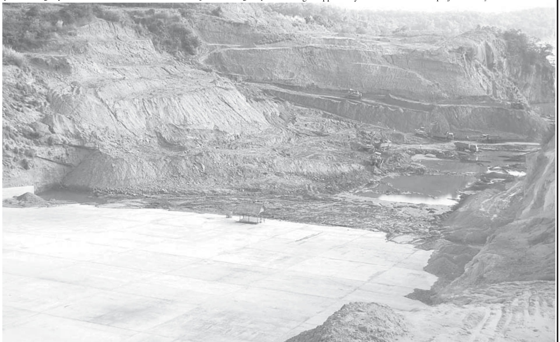
Kyeoohn-kyeewa Dam is under construction near Wunlo Village of Pwintbyu Township on 5 November 2008.
