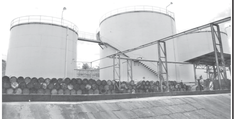
The 2000-ton palm oil tank and 500-ton palm kernel oil tank.
