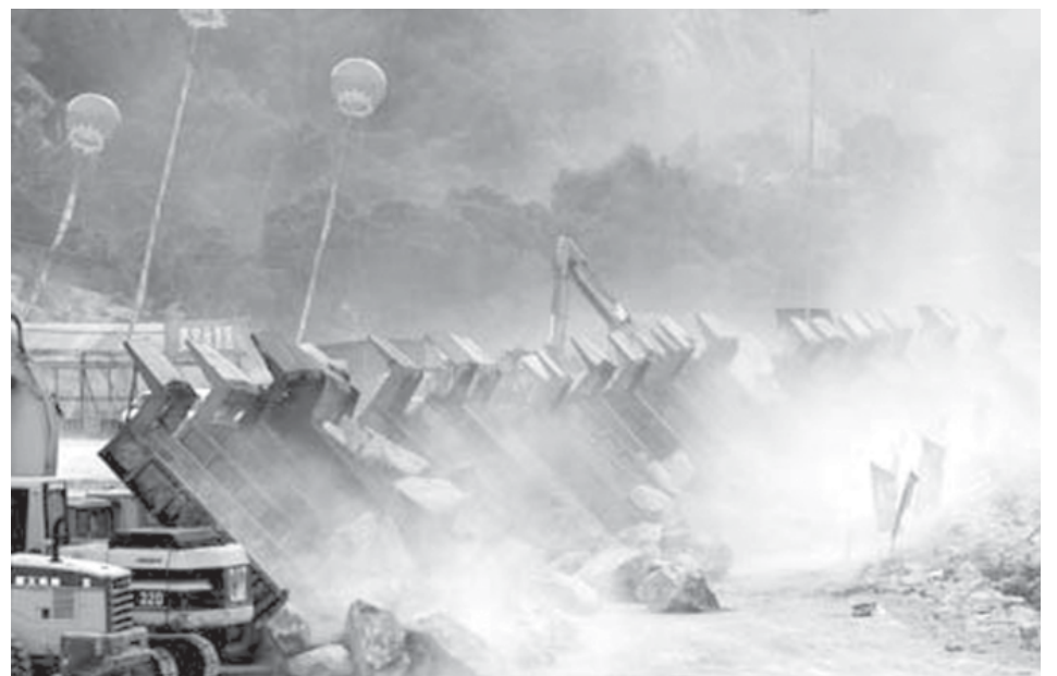
Lorries pour down earth at the construction site of the Nan'ao bridge during its groundbreaking ceremony in Nan'ao County, south China's Guangdong Province, on 20 Jan, 2009. The bridge of 11.08 kilometres across the sea will connect Nan'ao County, China's first 4A-class sea islet ecological tourist resort, with Shantou, a city also in Guangdong.—XINHUA
