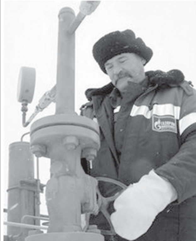
A technician inspects pipeline equipment and gas pressure at the gas metering station in Pisarevka, Russia, on the border with Ukraine, on 20 Jan, 2009. Russian natural gas began flowing on Tuesday into Ukraine after a nearly two-week cutoff that left large parts of Europe cold and dark and underscored the continent's vulnerability and dependence on Russia's energy.—INTERNET
