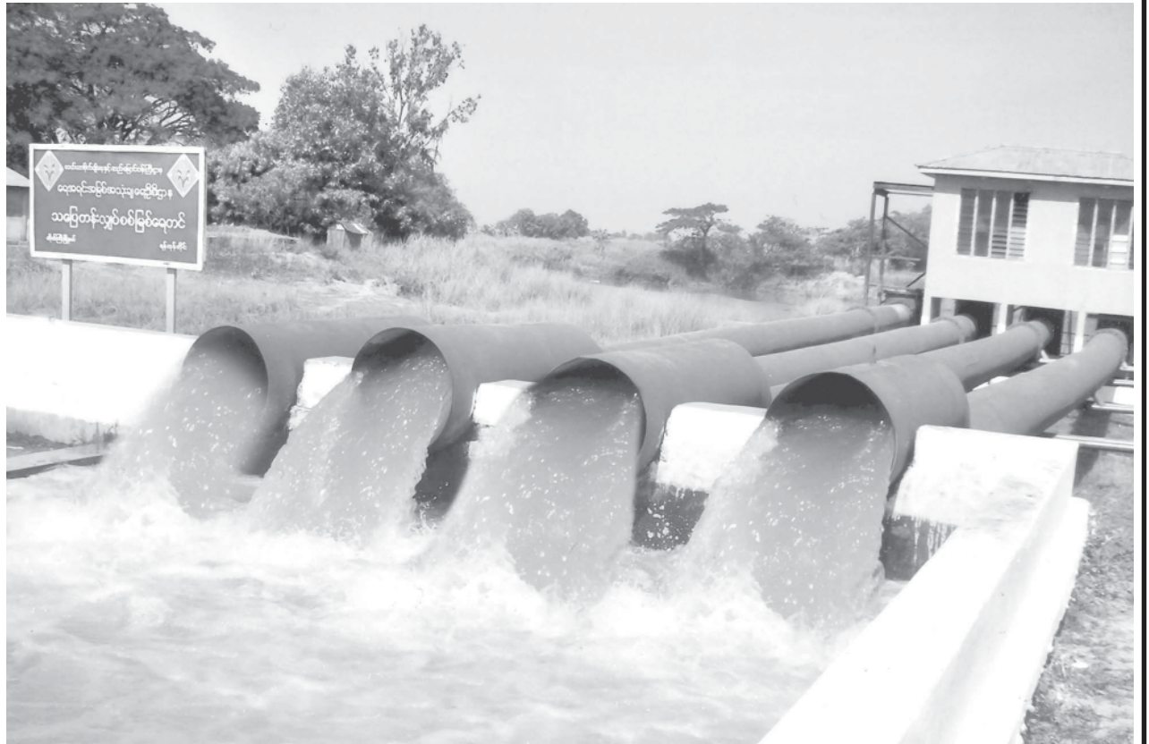
Thabyetan river water pumping station supplying water from Hline River to farmlands through main canal.
