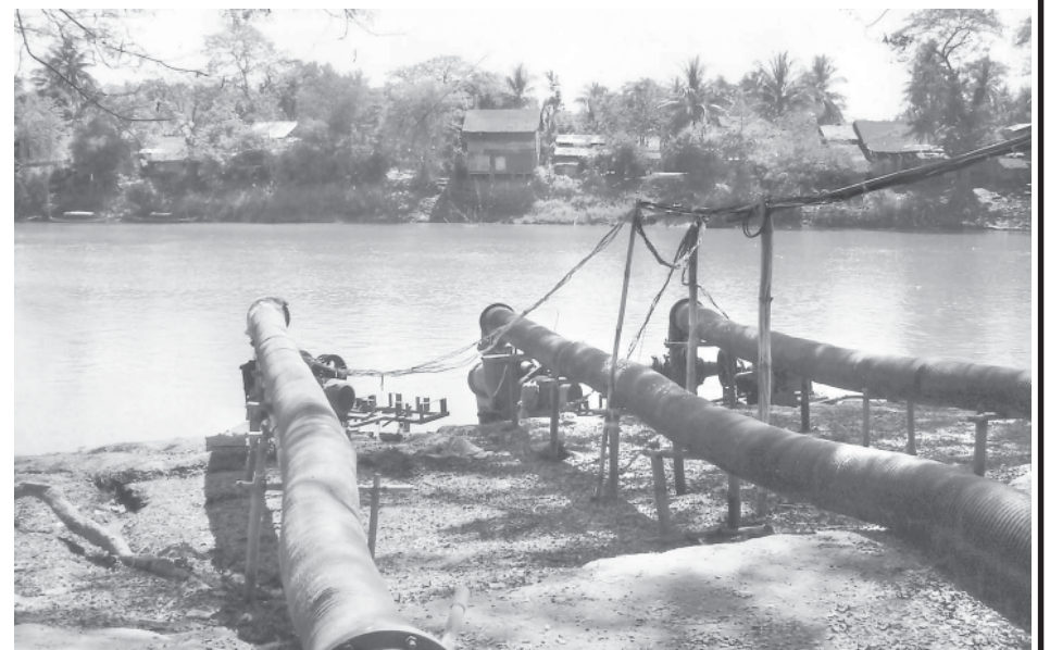
Taungyat Zigon river water pumping station installed with water pump and pipes to use water from Hline River.
