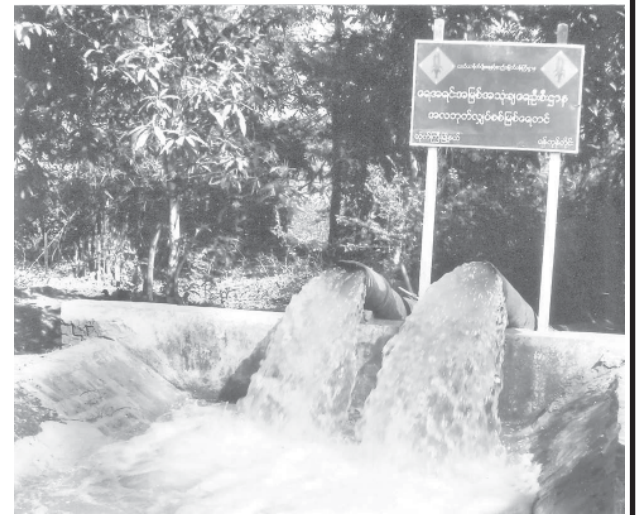
Water being pumped into main canal at Alabok river water pumping station.
