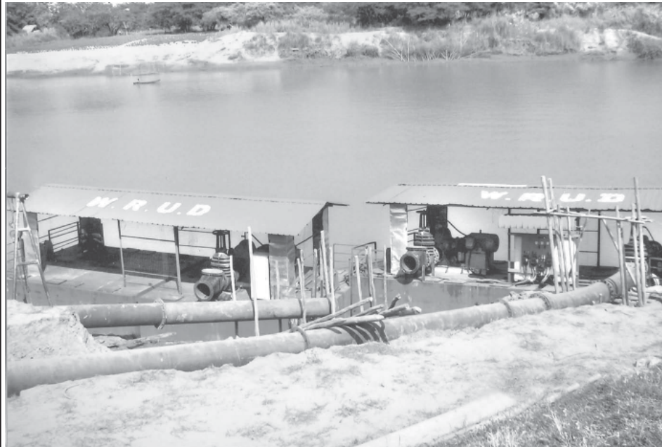
Aingkalaung river water pumping station pumping up water from Hline River by water pump and pipes.
