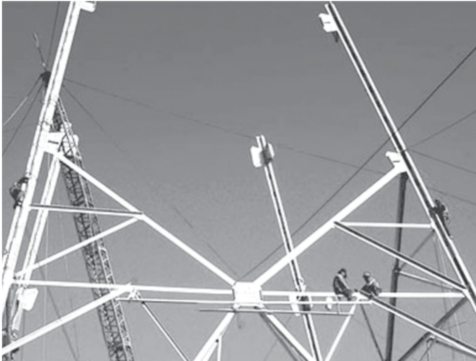
Construction workers erect a tower for an ultra-high voltage power transmission line from Baiyin to Yongdeng in Gansu Province in Northwest China.—XINHUA
