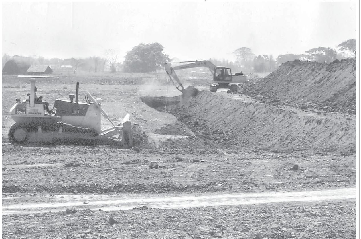
A bulldozer and an excavator carrying groundwork at Kayan Creek Water Pumping Project.
