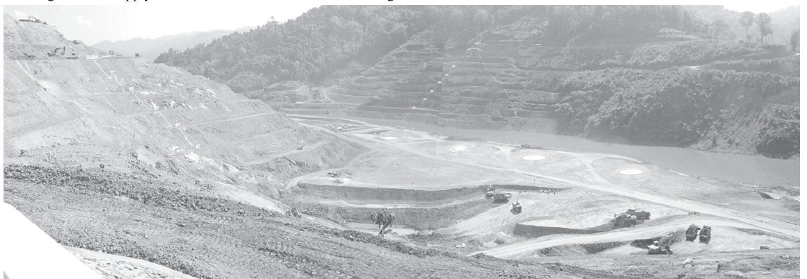
Thahtay Creek hydropower project in Rakhine State.—MNA
