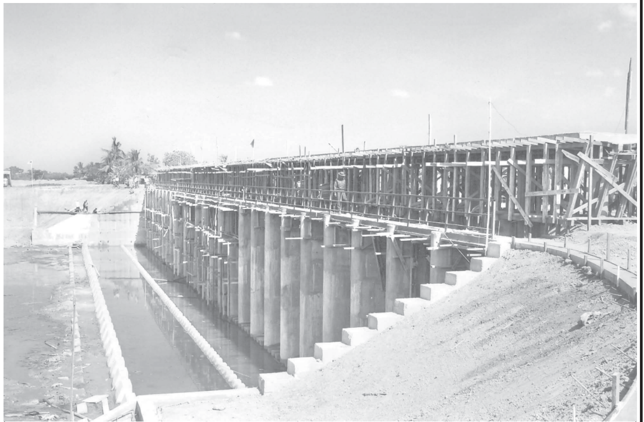
Kadappana Sluice Gate Project being undertaken by the Irrigation Department on the Kadappana Creek near Kadappana Village in Kyauktan Township.
