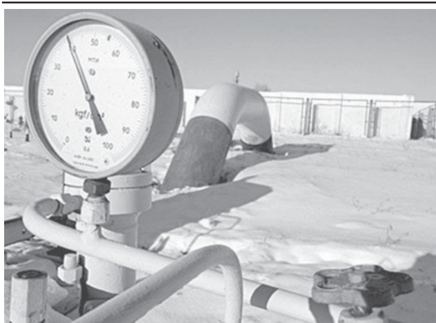
A pressure-gauge and valve are seen in front of a gas pipe at the gas-compressor station in the small Ukrainian city of Boyarka, near Kiev.
