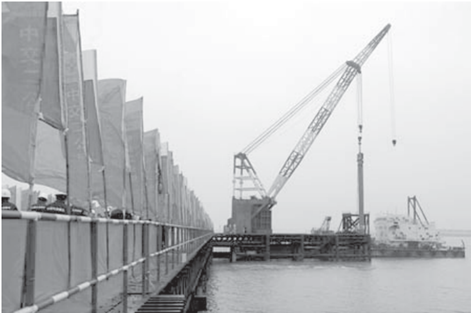
A crane drive piles as the construction of the No 4 Cross Yangtze River Bridge started in Nanjing, capital of east China's Jiangsu Province, on 28 Dec, 2008. The 28.996-km-long bridge has a span of 5.448 km, the longest in China and the third longest in the world. The No 4 bridge is scheduled to be completed in 2010 and put into operation in 2013. —XINHUA
