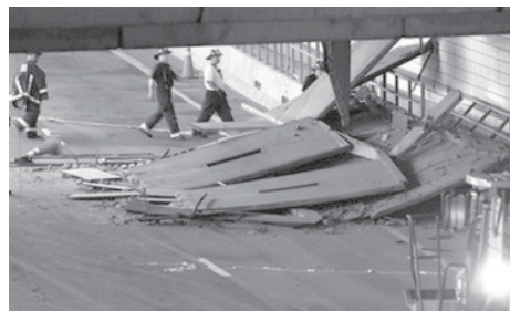
In this 11 July, 2006, file photo, firefighters inspect a section of ceiling in the Interstate 90 eastbound connector tunnel through Boston that collapsed onto the roadway and killed a woman passenger in a car.—INTERNET
