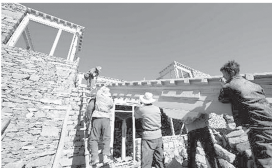
Farmers build a house in Gonggar County of Shannan Prefecture, southwest China’s Tibet Autonomous Region, on 9 Dec, 2008. —XINHUA
