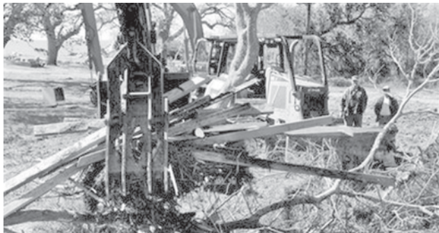
Workers watch as a back hoe drop a scoop of hurricane debris, on 25 Nov, 2008, in Smith Point, Texas. Spotters watch for bodies and hazardous debris as each scoop is lifted and moved.—INTERNET
