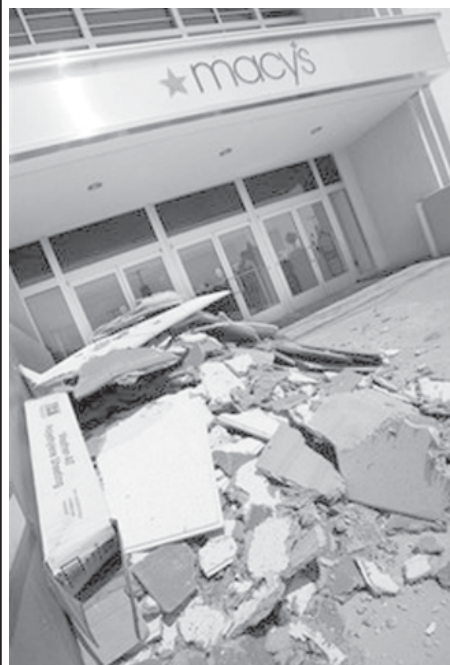
In this photo, ceiling tiles and other debris are piled outside, after pipes broke at a Macy's department store in the Canoga Park area of Los Angeles following an earthquake that rolled through Southern California.
