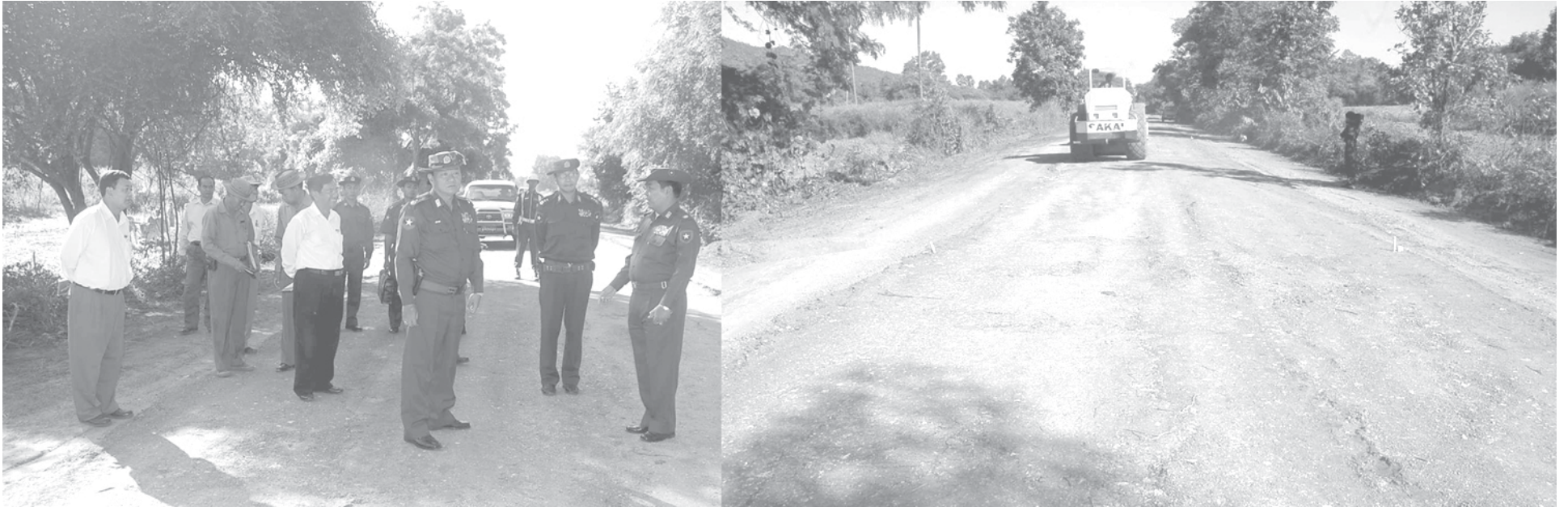
Maj-Gen Khin Zaw of Ministry of Defence inspects construction of railroad along Thayet-Pwintbyu road section.—MNA
