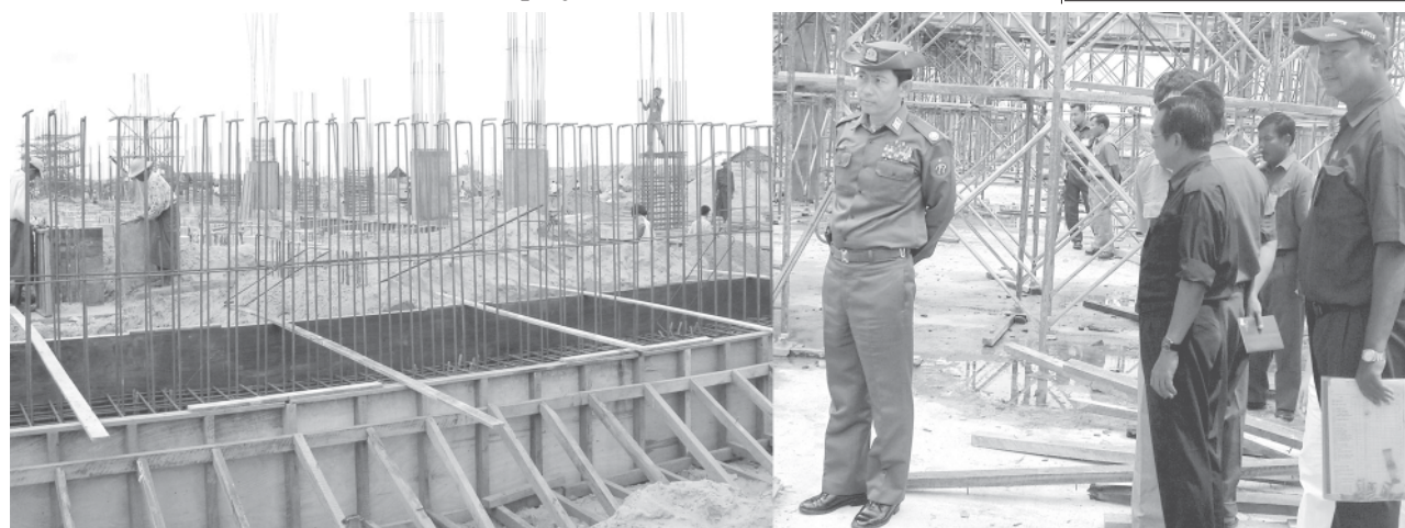
Deputy Minister Brig-Gen Than Htay inspects construction of Fertilizer Factory No. 4 in Hmawby. — MNA
