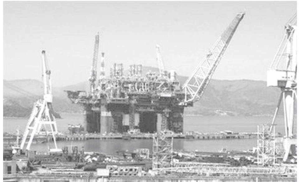
Photo shows a view of a Petrobras off-shore oil platform under construction in Angra dos Reis, near Rio de Janeiro. Brazil has inked a multi-million-dollar deal to explore for oil off the Cuban coast, joining India, Vietnam, Malaysia Spain, Norway and Venezuela in cash-strapped communist Cuba's quest for black gold.—INTERNET
