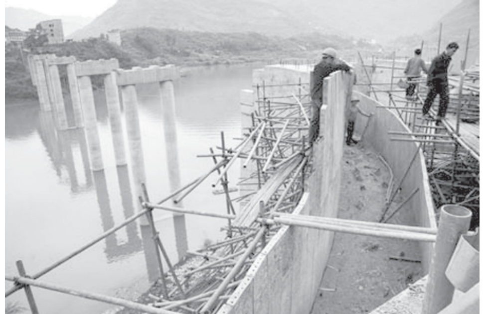
Workers build the new Nanxi bridge in Yunyang county, southwest China’s Chongqing Municipality, on 28 Oct, 2008. —XINHUA
