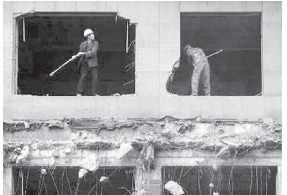
Workers demolish a building in Suining, Sichuan Province on 23 Oct, 2008. China's Ministry of Finance on Wednesday announced a series of policy changes that will make it easier for people to buy their first homes, fleshing out a directive approved last week by the cabinet.— INTERNET
