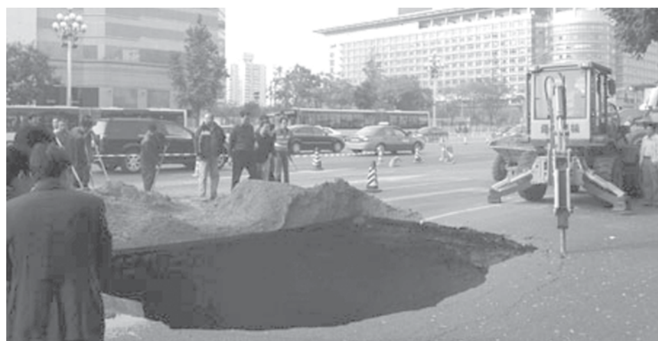
Workers repair West Chang'an Avenue in Beijing, capital of China, on 17 Oct, 2008. Chang'an Avenue collapsed on Friday. —XINHUA
