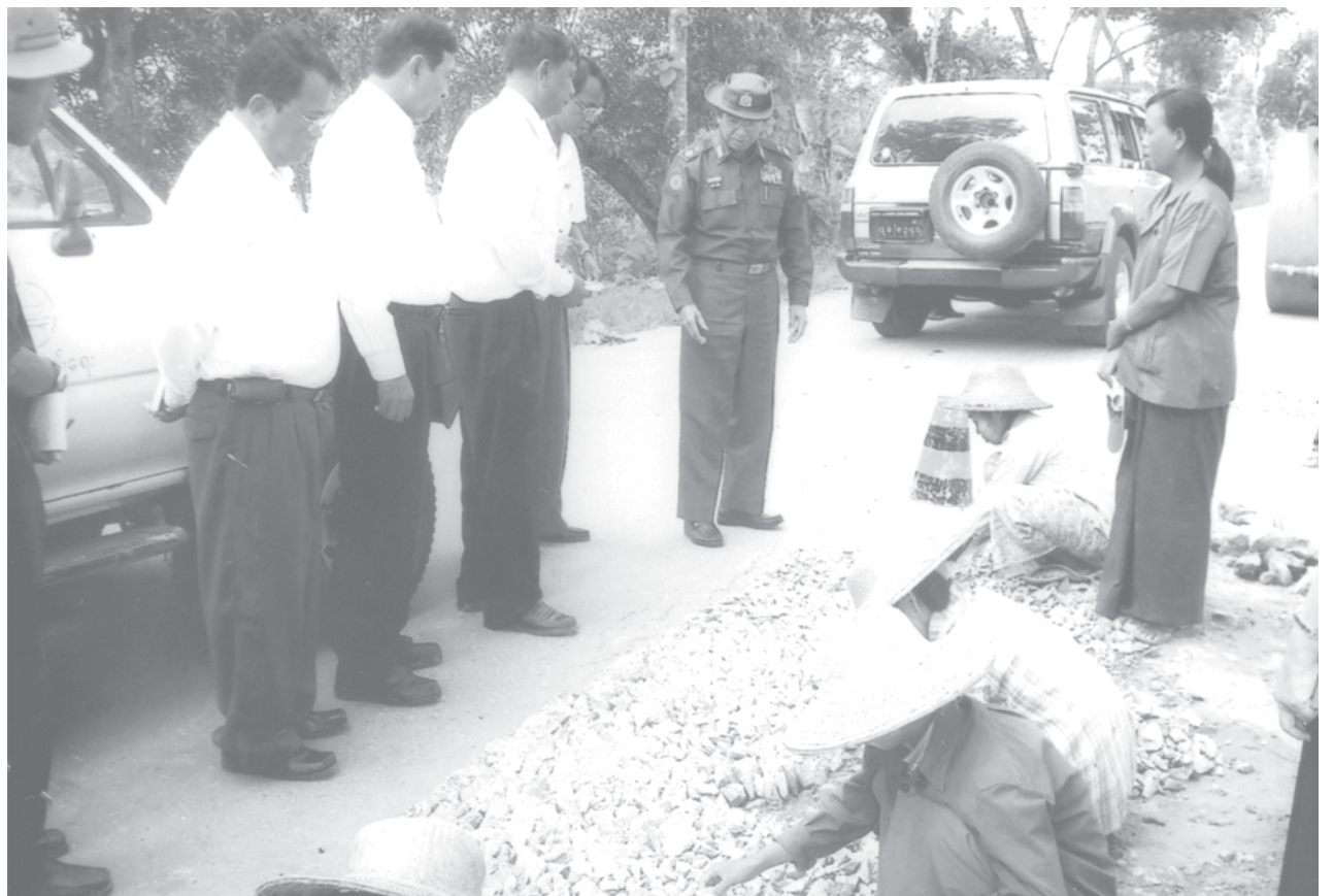
Minister for Construction Maj-Gen Saw Tun inspects maintenance of Yangon-Pathein Road. CONSTRUCTION
