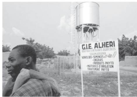
A water tower that is filled using energy from solar panels near Maradi in Niger. With an average daily dose of five-to-seven kilowatts per hour (kWh) for every square metre (10 square feet), Africa has more potential for producing energy from the sun than almost anywhere on Earth.—INTERNET
