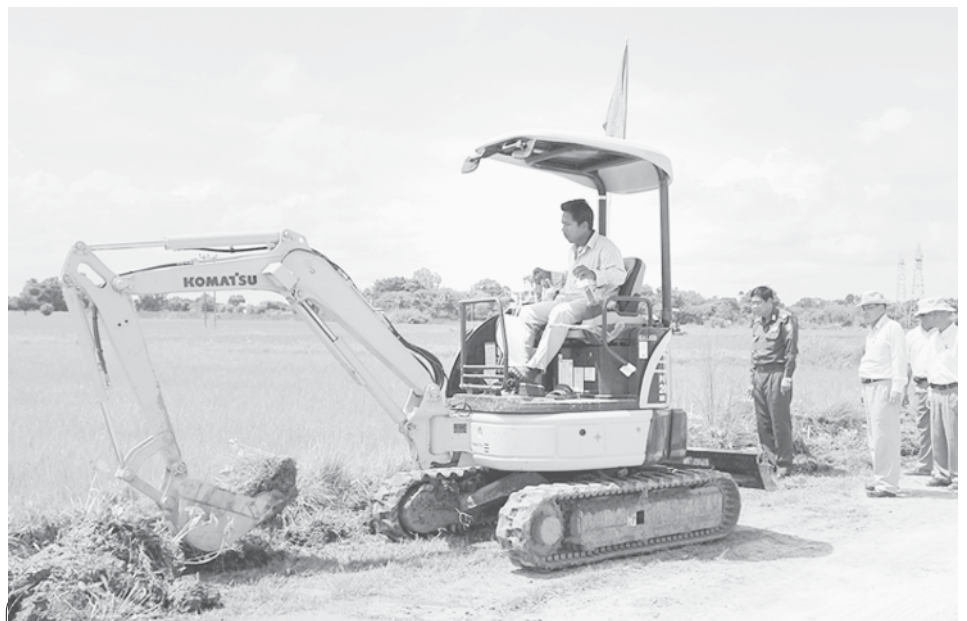
Minister Maj-Gen Htay Oo inspects dredging of canal at Minye Dam in Kyaukse.—A&I
