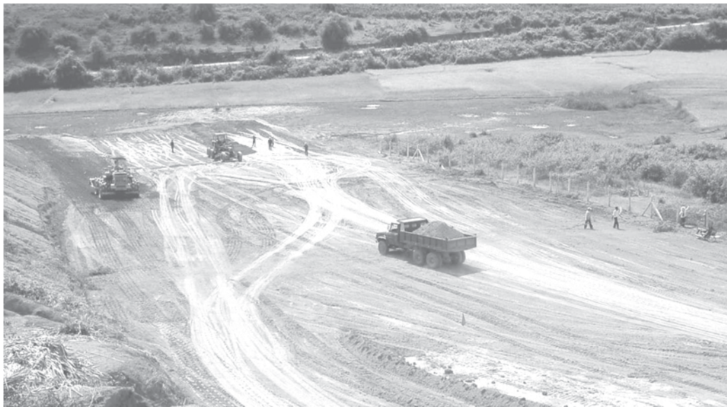
Maj-Gen Min Aung Hlaing of Ministry of Defence looks into runway extension project of Kengtung airport.—MNA
