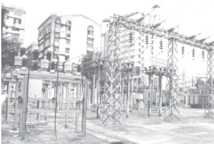
Minister for Electric Power No. 2 Maj-Gen Khin Maung Myint at a subpower station in Mayangon.—MNA
