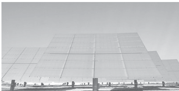
A solar thermal electric power plant in Sanlucar La Mayor in February 2008. The world must speed up the deployment of solar power as it has the potential to meet all the world's energy needs, the chairman of an industry gathering which wrapped up Friday in Spain said.—INTERNET
