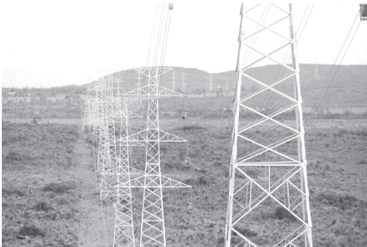
Nawnghkio detour power line of Mansan-Shwesaryan section.
