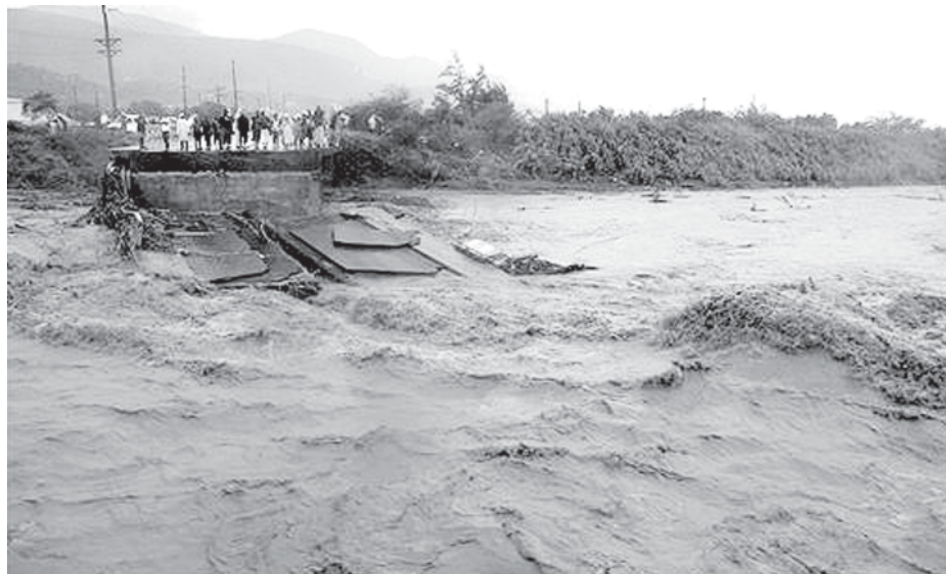
Residents watch a bridge that collapsed due to heavy rains caused by Tropical Storm Gustav in Kingston, Jamaica, on 29 Aug, 2008. Gustav ripped off roofs, downed power lines and pounded rain into Jamaica, triggering landslides and flooding but no reported deaths. —INTERNET
