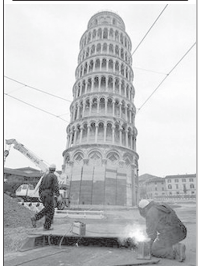
Workers are pictured at the base of the leaning tower of Pisa. (News on page 5)
