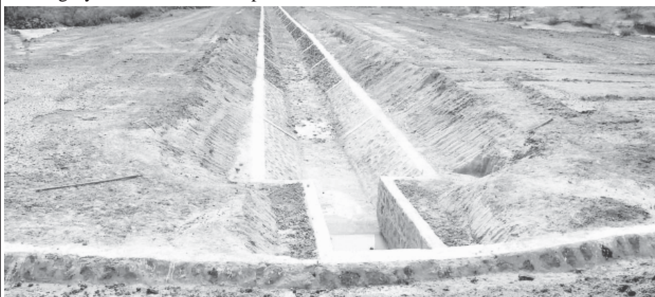
The main canal that will irrigate 150 acres of farmlands in Myaing Township.
