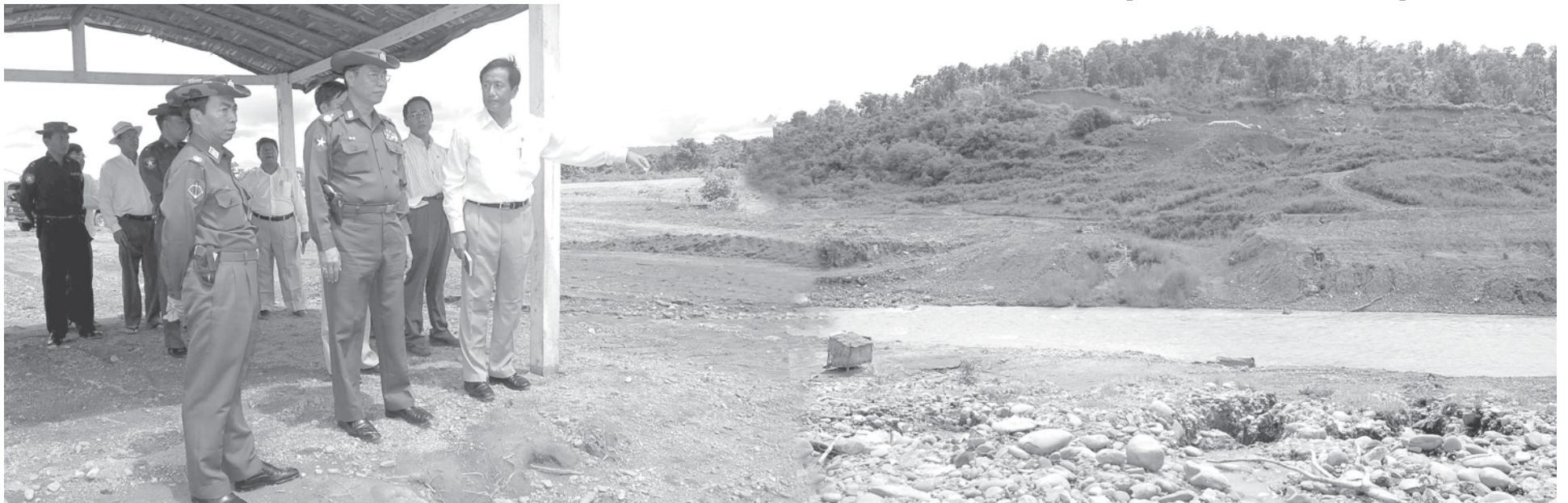
Maj-Gen Ohn Myint of Ministry of Defence looks into earth work of Yazagyo Multi-purpose Dam Project in Kalay Township.— MNA
